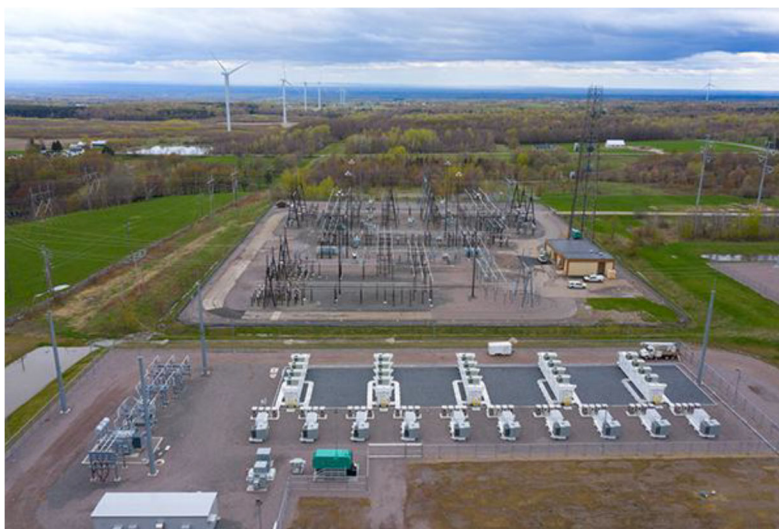
Figure 5-5: Northern New York Energy Storage Project (Sky view)
