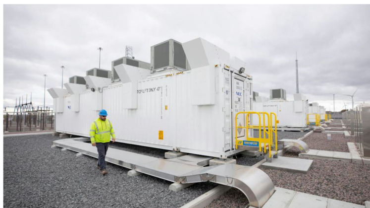
Figure 5-6: Northern New York Energy Storage Project (Ground view) 142
