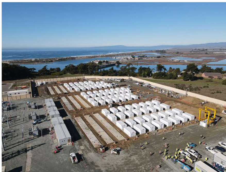
Figure 5-7: Moss Landing Energy Storage Facility 177
