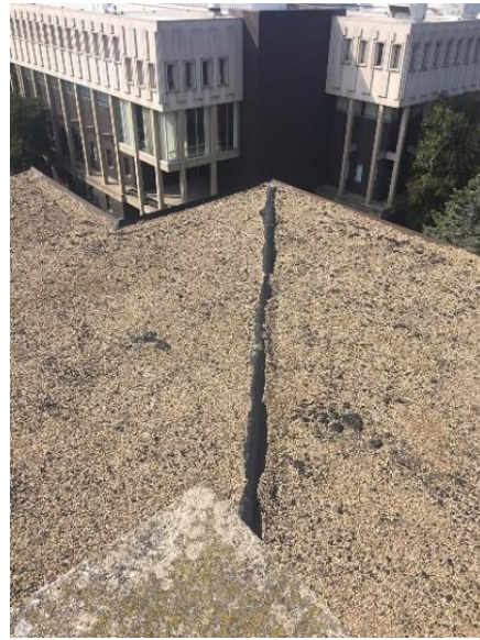
Water infiltration on roof
