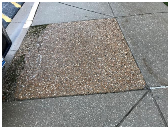
Crumbling wheelchair ramp
