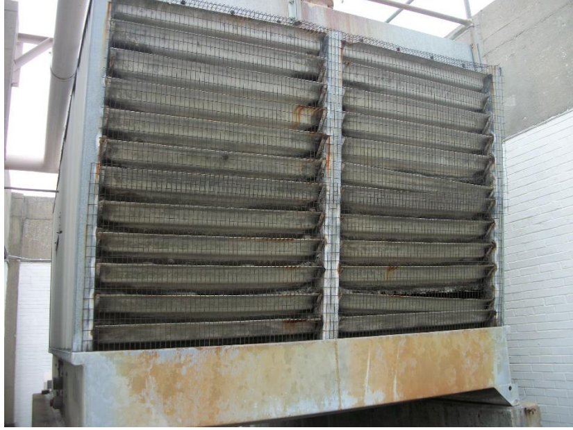
Corroded cooling tower
