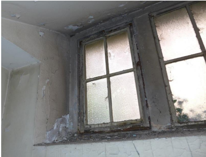
Window and drywall damage
