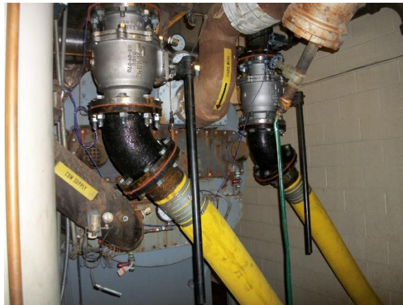
Temporary chiller hook up
