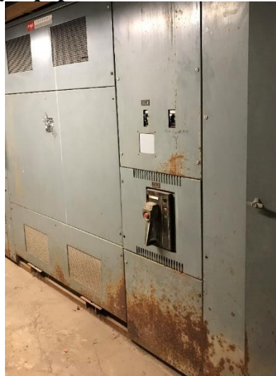
Switchgear from the 1960s
