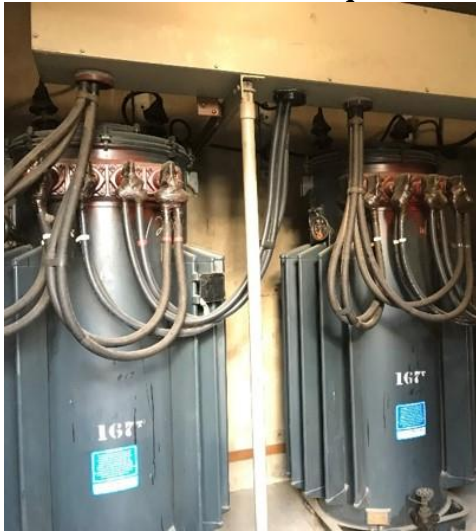
Transformer from the 1950s (with exposed live copper)
