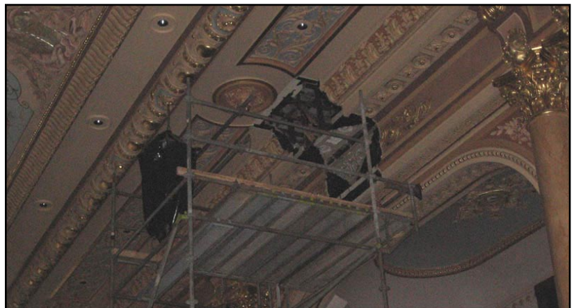
Plaster patch where ceiling speaker was removed.
